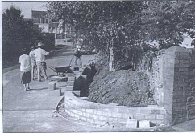
Going up: The wall being built over the verge on the approach road to St Bonaventure's Primary School
